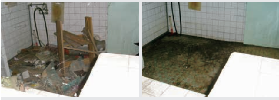
防火巷淨空執行前後對照 Before and after of clearance of fire safety alleys
